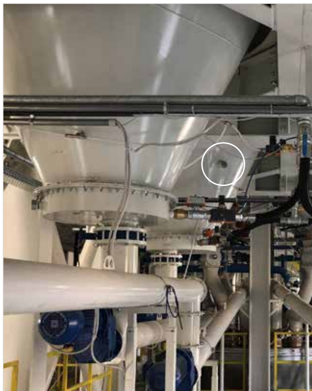
VBS (aeratori) - Silos
